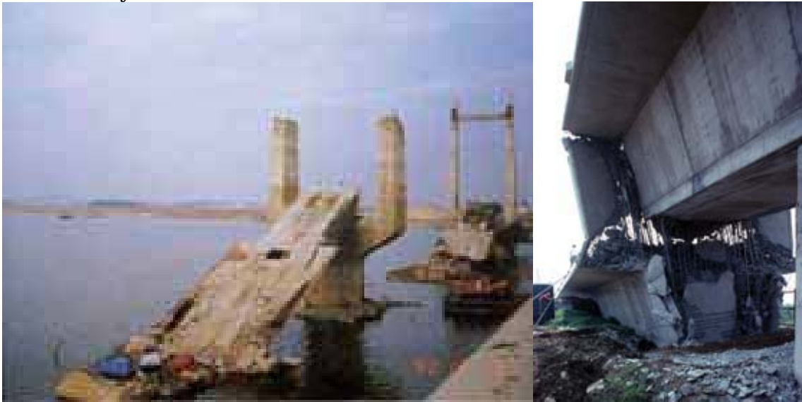
Photograph 1 the situation right after the collapse accident of New Haengju Bridge. (Donation: Prof.Yozo Fujino, University of Tokyo)
