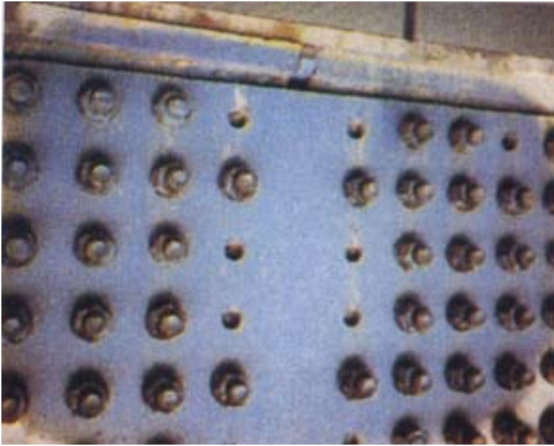
Photograph-2: Bolted joint minute of the splice plate (there is a position where the bolt has not been installed. (Source: Nikkei construction))
