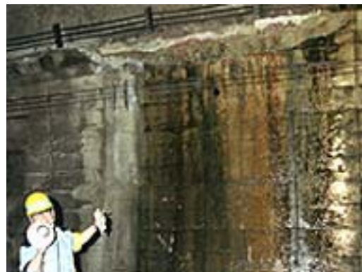
Figure 1. Kitakyushu tunnel flaking site
