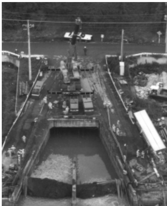
Figure 2 the aspect of the site on the day after the accident (September 20th, 1991)
