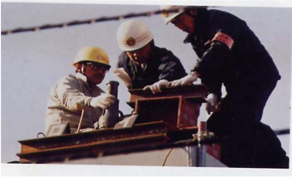
Picture 3: the H-beams which lack reinforced ribs (source : "Construction Accident" (Nikkei Construction) p16)
